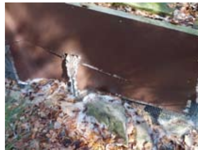
...and the aluminum flashing.
