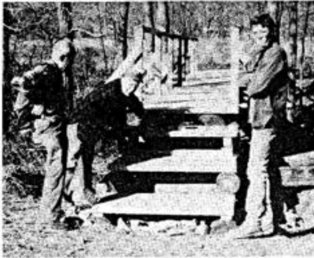
L/R: Thurston Griggs, Paul Ives, Kevin McGraw inspecting steps they built onto a footbridge along Conodoguinet Creek, Cumberland Valley PA, Appalachian Trail construction, 11/24/90. Photo by Ted Sanderson.
